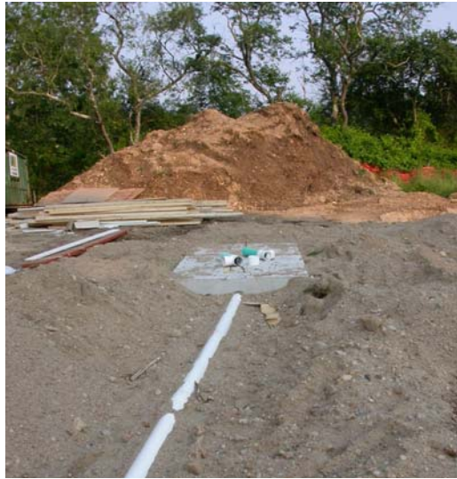
Figure 2: Septic Tank (Residential)
