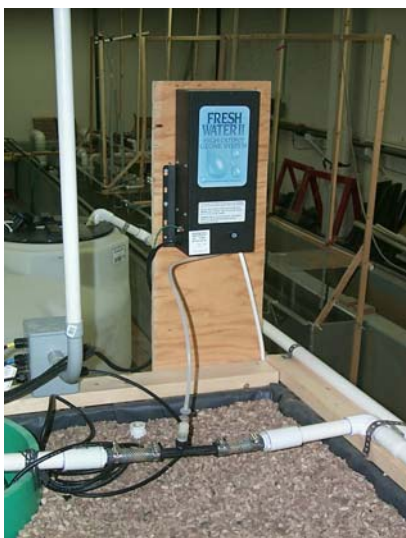
Figure 15 Spa Ozonator Used for Wastewater Disinfection
