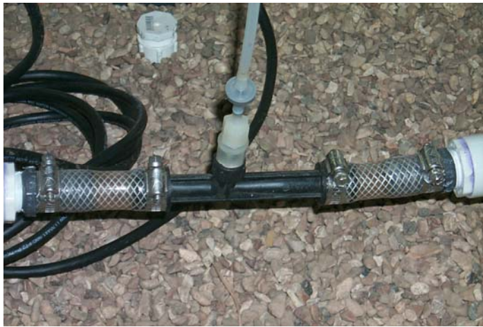
Figure 16 Venturi for Ozone Injection into Treated Wastewater
