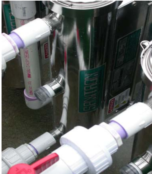
Figure10 Ultraviolet Disinfection Unit (Single Unit)
