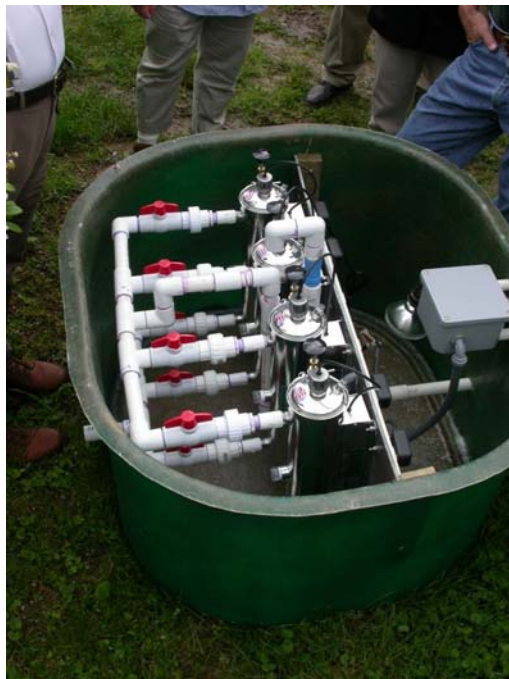
Figure11 Ultraviolet Disinfection System
