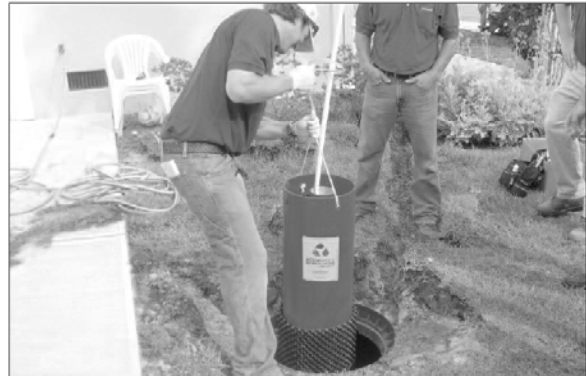
Typical Remediator Installation
